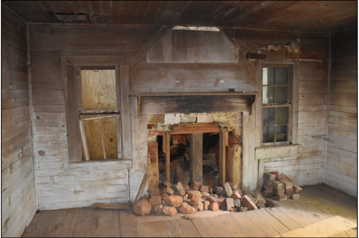
Figure 191- Inside the north room of the purported slave quarters/Reuben Jones House, facing north towards the covered windows and crumbling fireplace of the north elevation.
