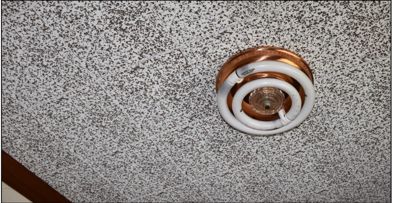
Figure 141- Non-original asbestos-containing ceiling tiles in the storage room just north of, and accessed from, the west room (see site plan in figure 122).
