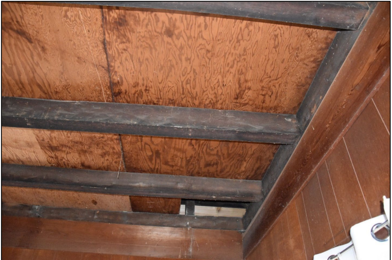
Figure 183- Looking up at the ceiling of the kitchen/schoolhouse, with historic wood beams and non-historic plywood.
