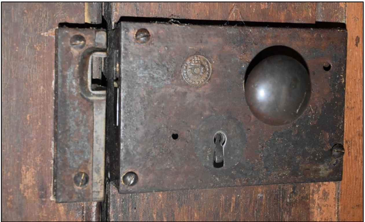
Figure 138- Detail of the circa mid-to-late 1800s door lock on the west room's exterior door; note the sailing ship emblem, and the flaking painted wood graining on the door itself.
