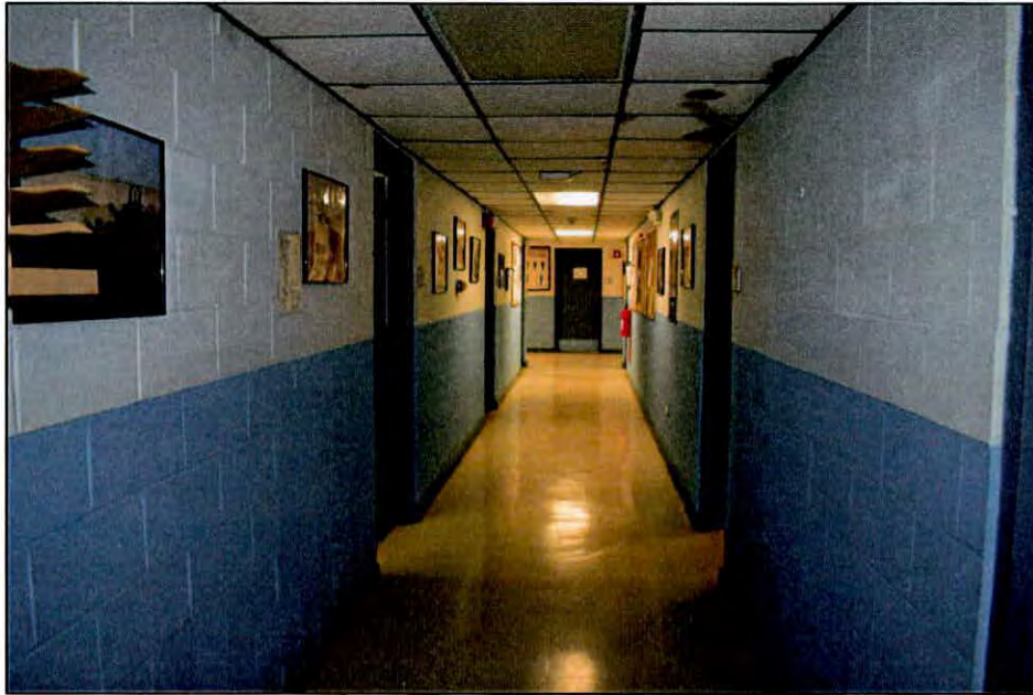
Figure 13.19. Corridor in the Whiteville Armory, exhibiting vinyl flooring and acoustic ceiling tiles with water damage.
