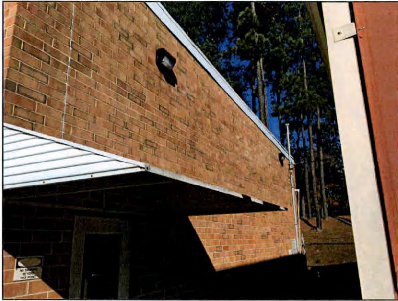
Figure 12.14. Exterior lighting of the Raleigh TMP at Raleigh Armory after replacement.
