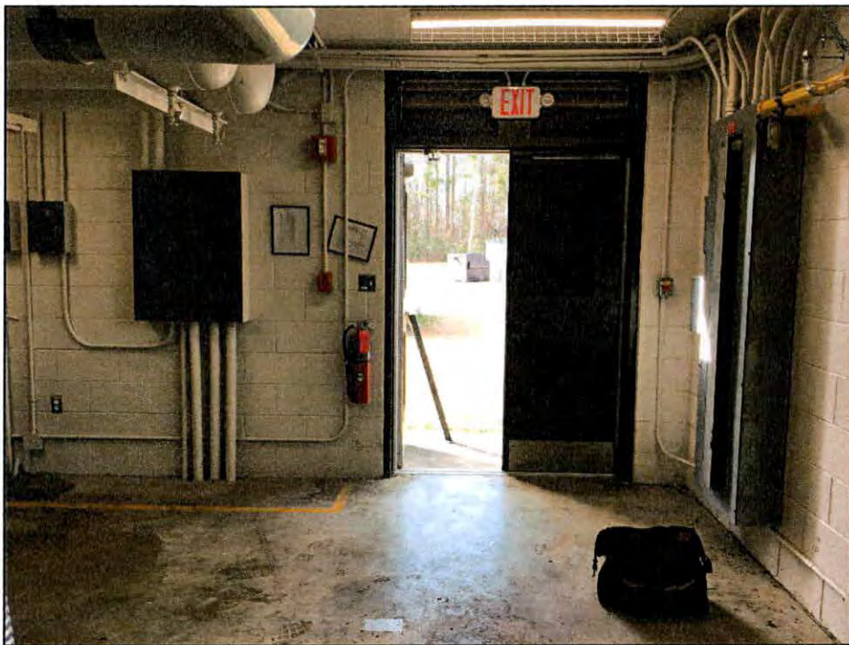
Photo 5.24. The boiler room at the Beulaville Armory.
