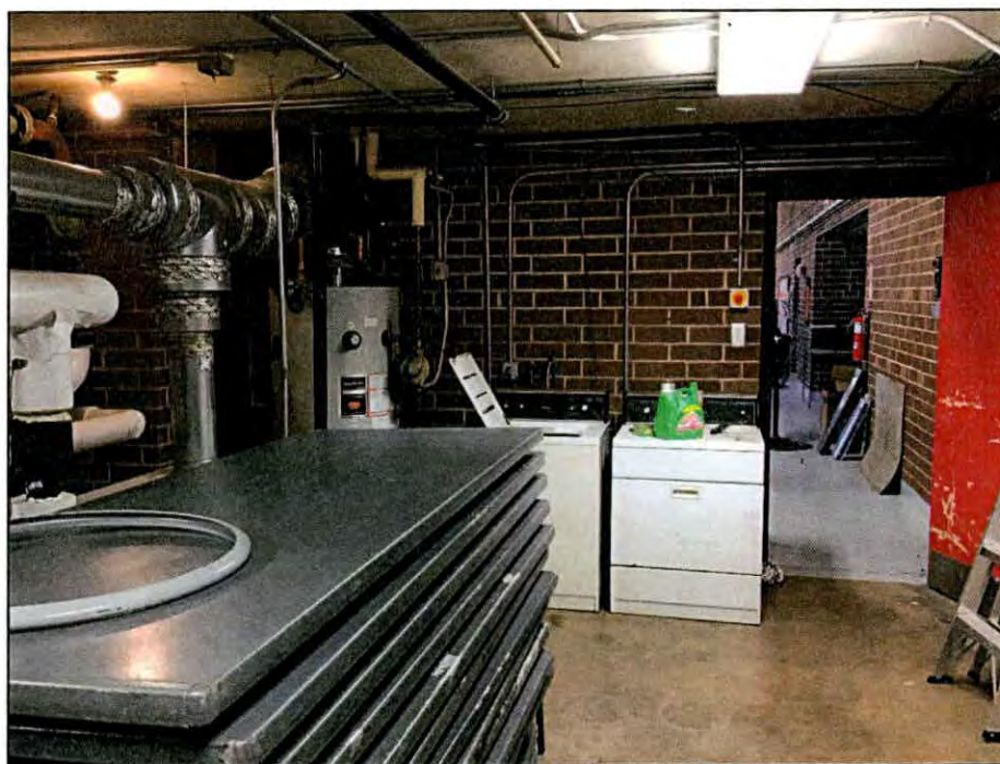
Figure 7.25. Boiler Room at the Butner Armory.
