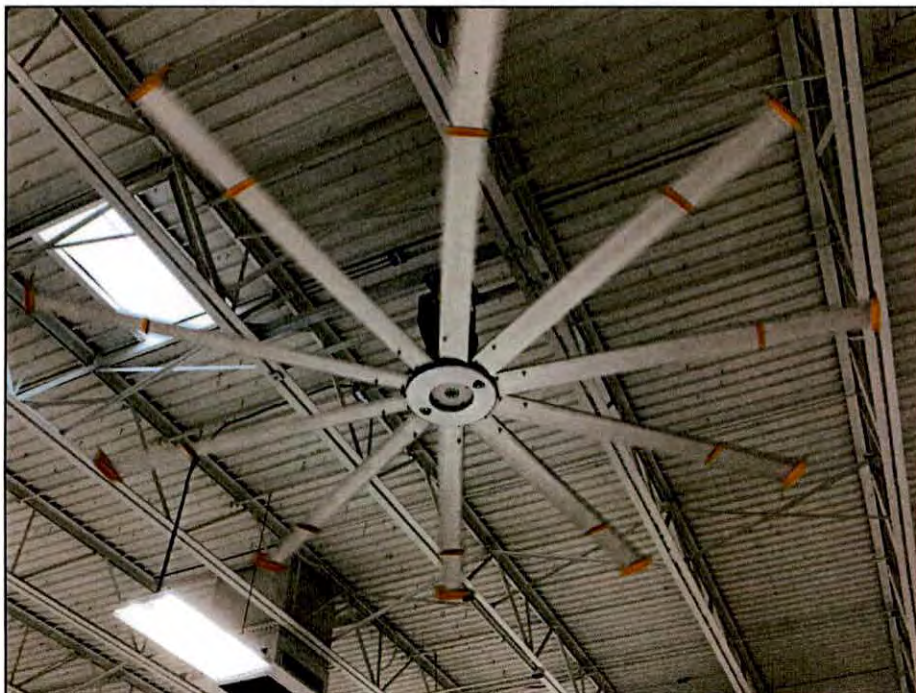
Figure 6.26. Representative large metal fan in the assembly hall at Boone Armory.
