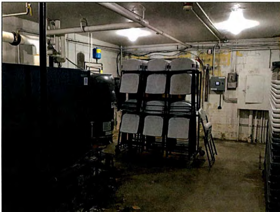
Figure 14.25. Boiler/storage room at the Youngsville Armory.
