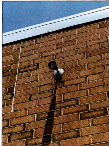
Figure 12.13. Exterior lighting of the Raleigh TMP at Raleigh Armory before replacement.
