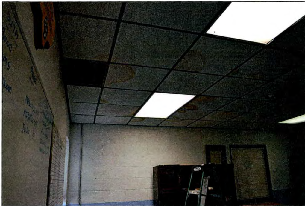
Figure 13.22. Water damage to acoustic ceiling tiles.
